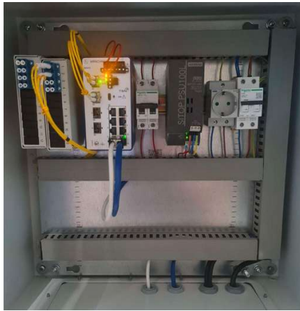
Figure 2. OT network electrical panels, housing the industrial switches and optical fiber ring terminations that support the plant's communication infrastructure.
